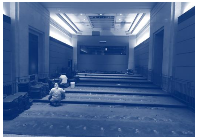
The Jesse H. Jones Theatre for Texas Studies closed for a week in September for scheduled repairs, including the removal of all seats, to allow inspection and repair of the raised flooring that provides a clear view of the front of the stage and screen. New seats and technical upgrades will also be installed, thanks to a grant from the Albert and Ethel Herzstein Charitable Foundation.
